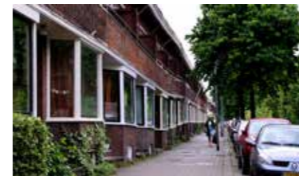
Funderingsproblemen Sagging foundations
